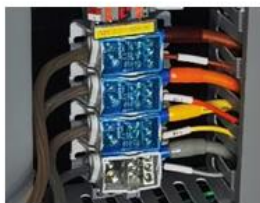
Auxiliary power input cable(L1/L2/L3/N)5AWG*4
