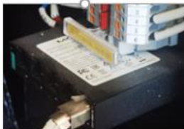
Network communication wires
