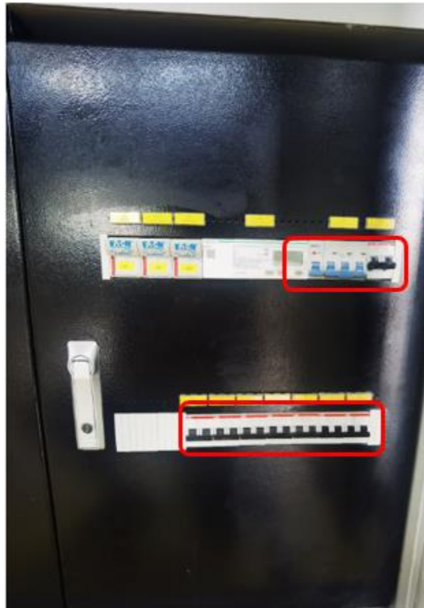
Figure 7.the position of the air switch
